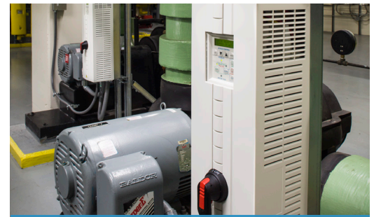
VFDs installed on chilled water pumps paid for themselves in energy savings in about a year.
