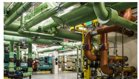
New VFDs, building automation and HVAC programming have helped drive down cooling costs.
