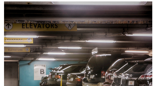
High-efficiency fixtures installed in the Summit Parking Deck qualified for more than $9,400 in rebates.
