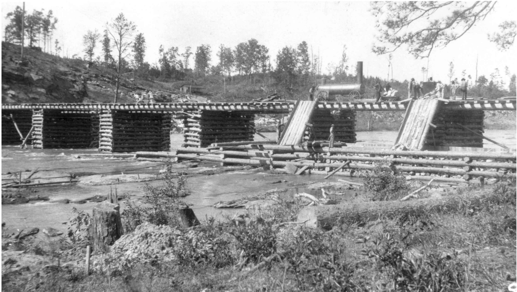
Figure 18. Detail View of Filling of Downstream Rock Filled Timber Crib Cofferdam Section
