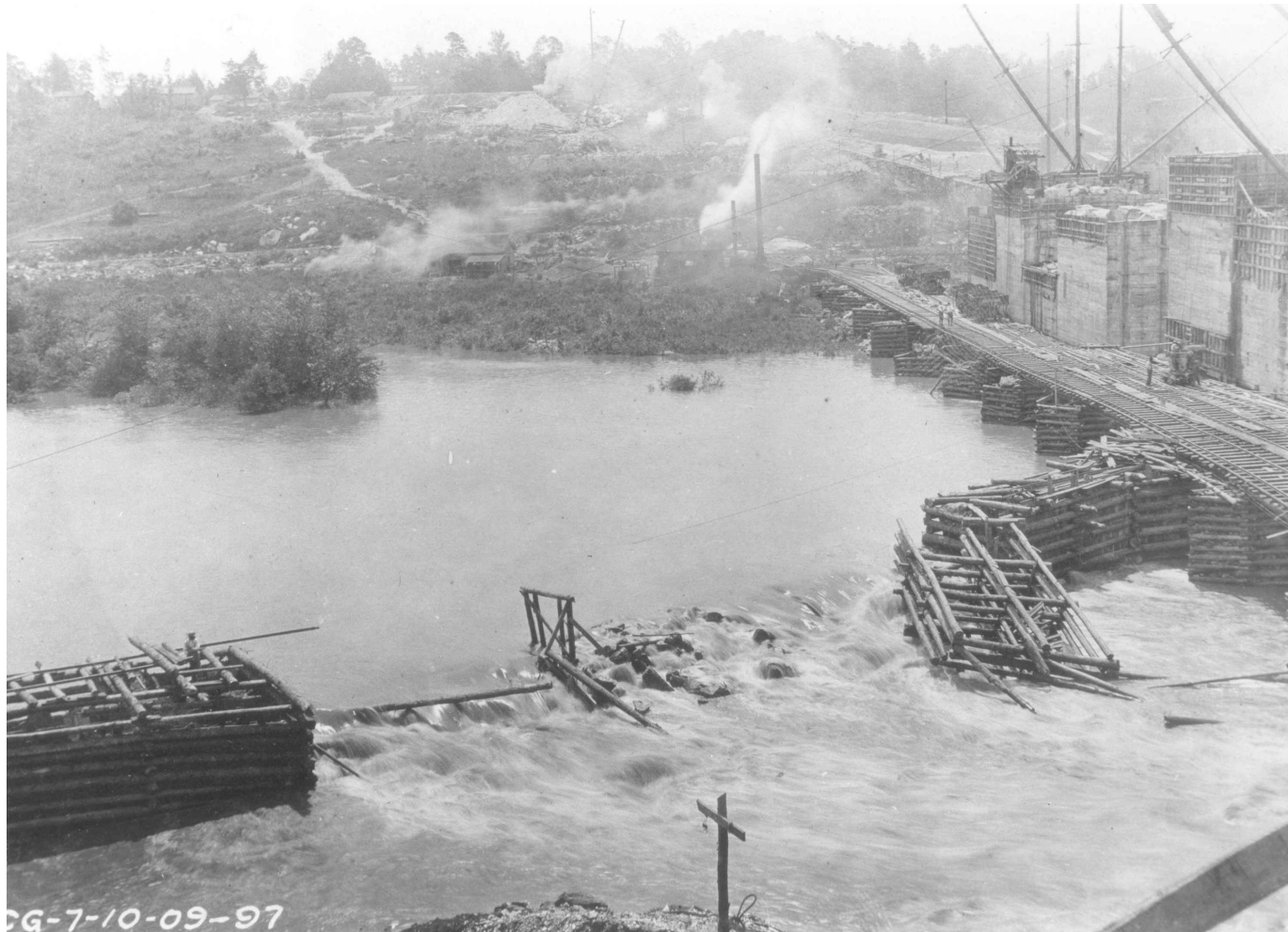
Figure 65. Second Cofferdam, Northwest-to-Southeast Cribwork Failure
