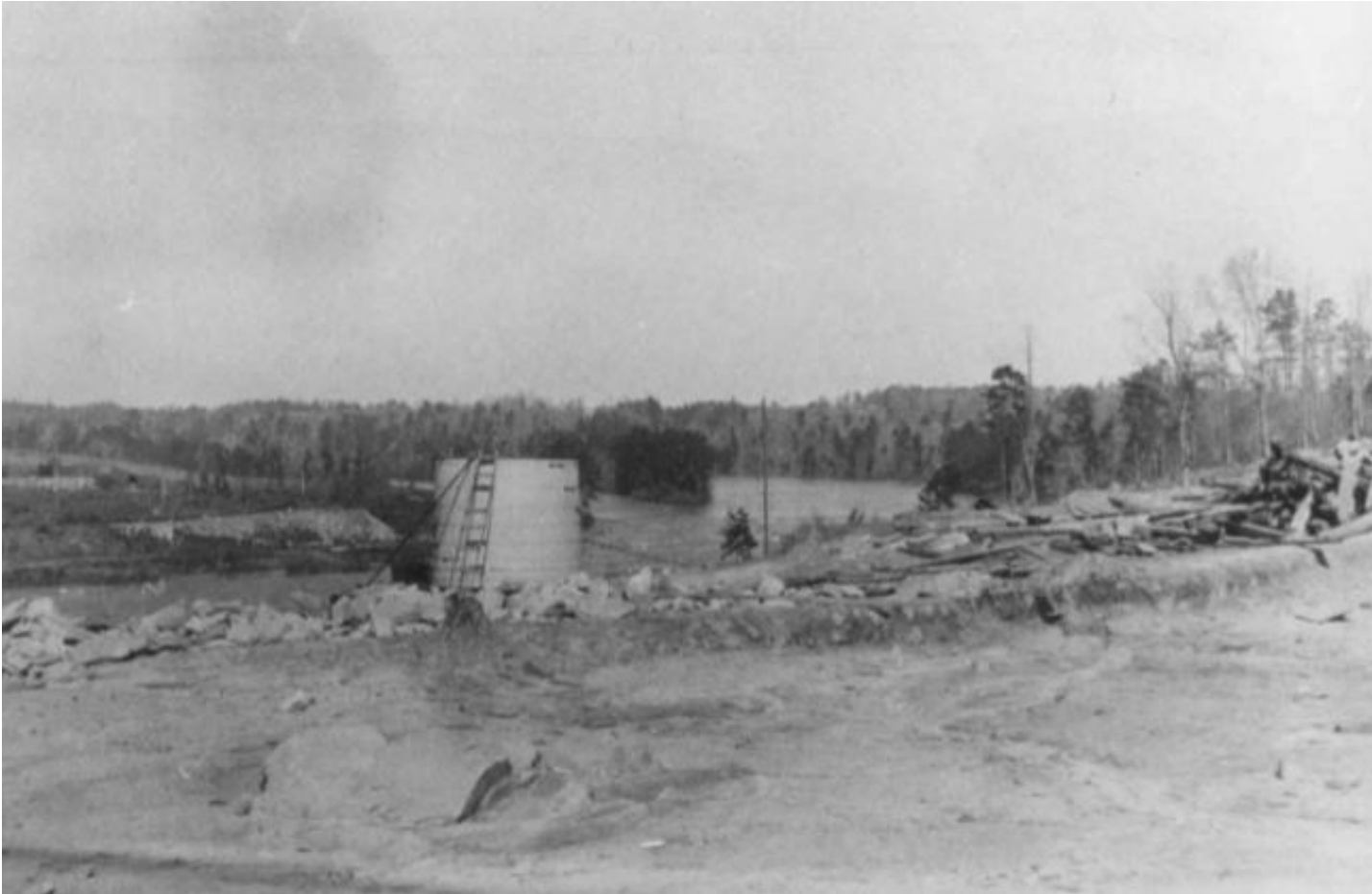
Figure 9. Water Storage Tank/Catchment
