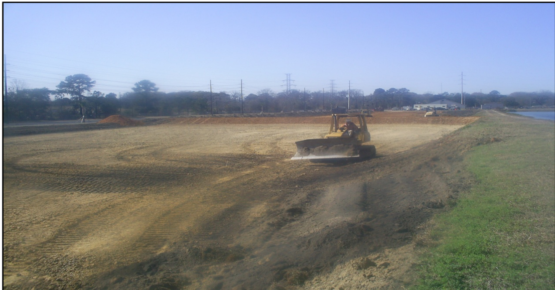
Expanded fuel tank secondary containment – note new clay berm in background
