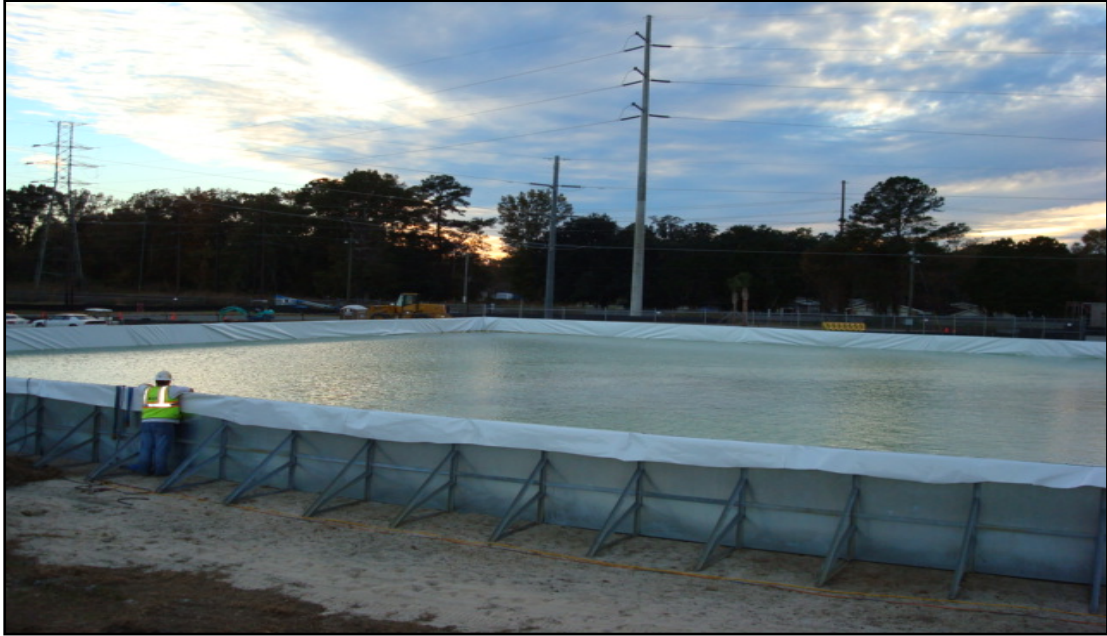
500,000 gallon temporary tank for water storage and treatment
