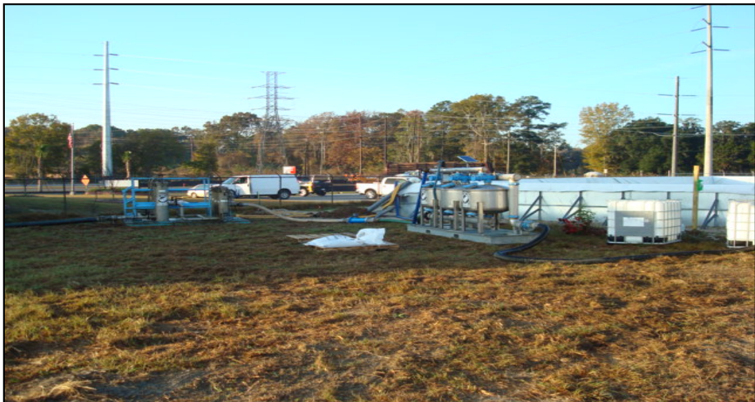
Water Treatment and filtration system
